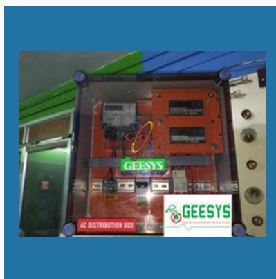
Solar ACDB Box
