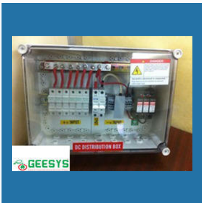
Solar Array Junction Box
