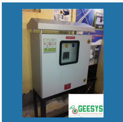
Solar AC Distribution Box
