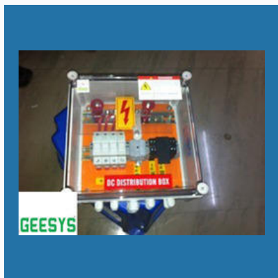
Solar Array Junction Box for 15kwp
