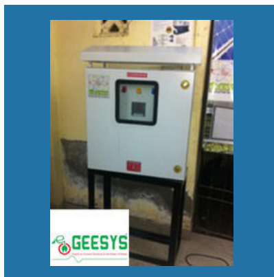
Solar AC Distribution Box
